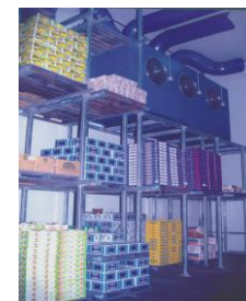
Storage technology and equipment
